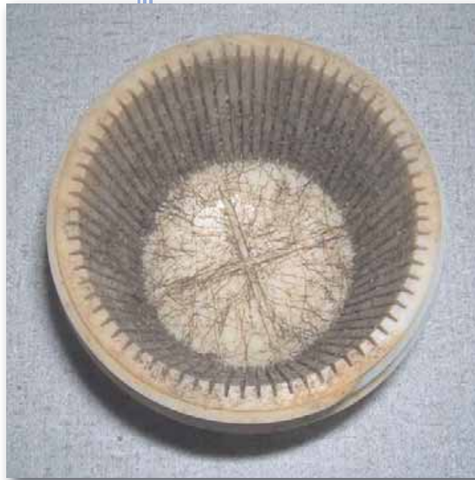
Before treatment – heavy colonisation of the under-drain nozzles and stems with hydroid Cordylophora (and zebra mussels in some cases) had reduced the filters' capacity
